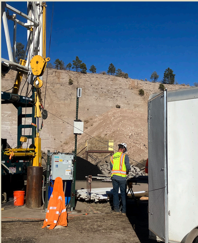
R-67 Well Maintenance
